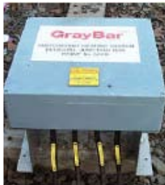
Wall Mounted Off Track Junction Box 0055/020814
