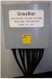
Post Mounted Off Track Junction Box 0055/021034
