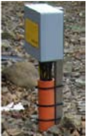
Post Mounted Off Track Junction Box 0055/020813
