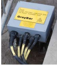
Base Mounted Off Track Junction Box 0055/021036
